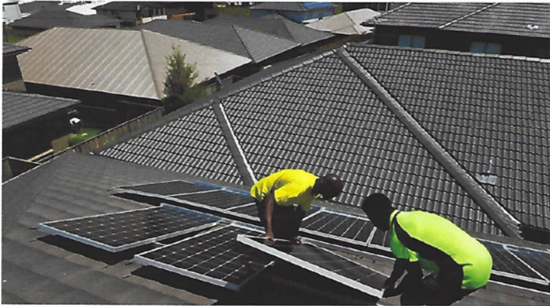
Lots more roofs to cover: Solar PV penetration rates still lag in Sydney and Melbourne. NICK MOIR
